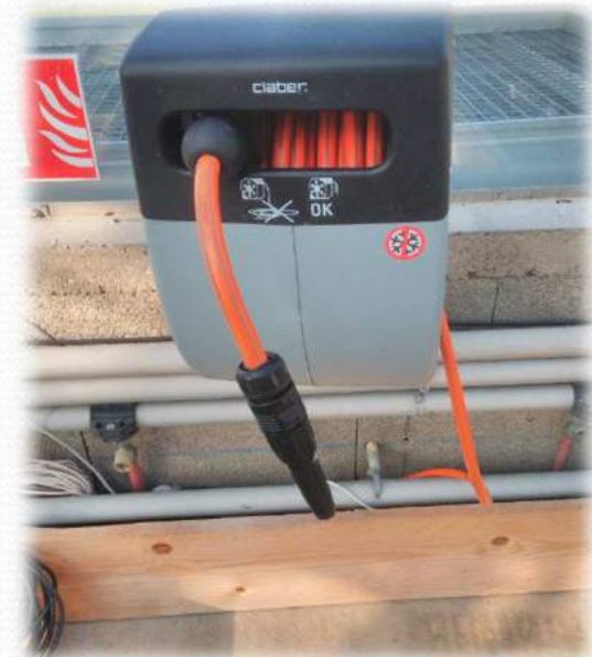
Tuyau de rinçage (bord des bassins)
